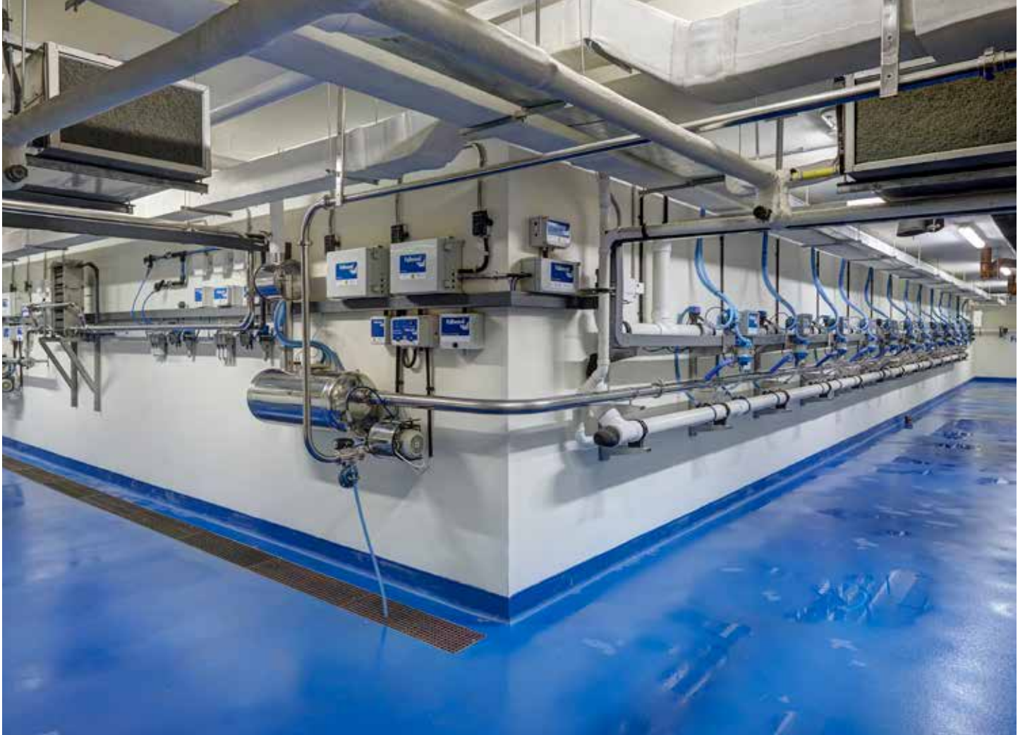
CELLAR MILKING SYSTEM
